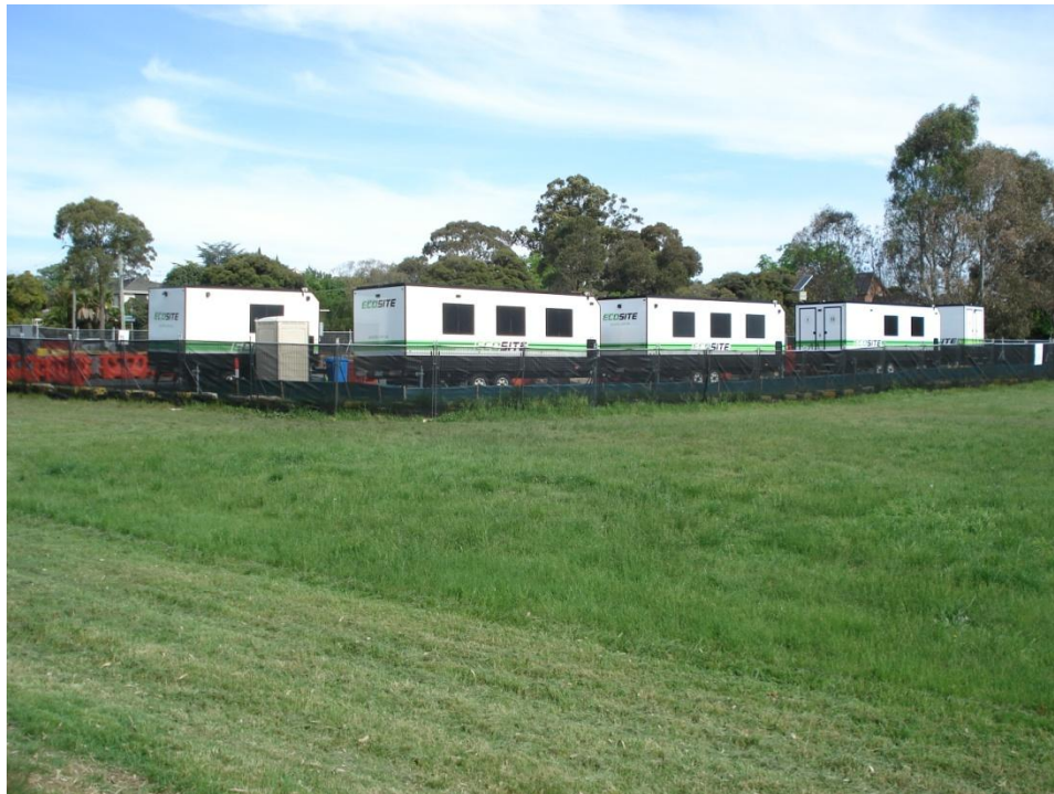
Photograph 14: Site compound near Kosciusko Road, Balwyn North with site sheds cynically labelled 'Eco Site'
