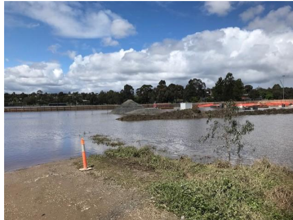
Photograph 1: North East Link Project early works site flooding, Marcellin College, Bulleen Road, Bulleen, November 2022.
